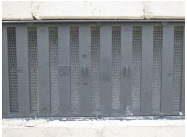
Concrete block prevents air flow into crawl space at foundation vent
