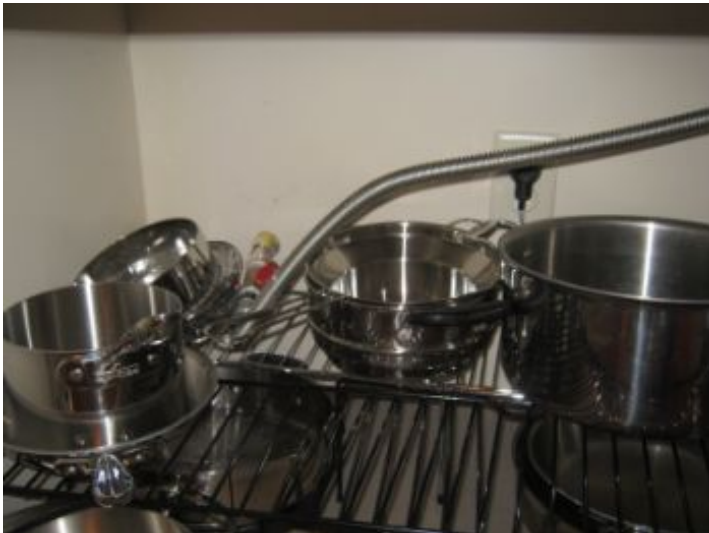
Gas piping beneath range does not appear to be properly protected from physical damage
