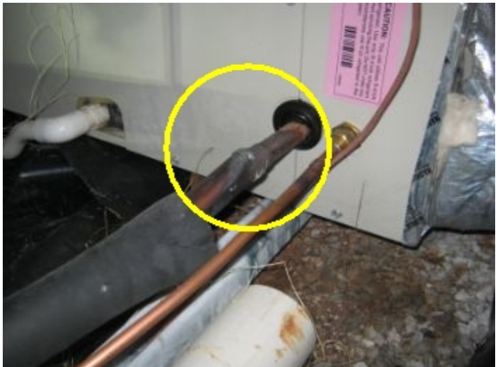
Cooling system refrigerant lines need insulation - Sections of the insulation on the compressor lines appear to be missing. These lines should be suitably insulated for the proper operation of the compressor.
