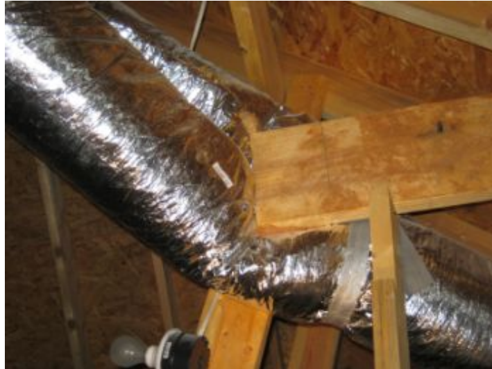
Flex duct observed in a bind in attic
