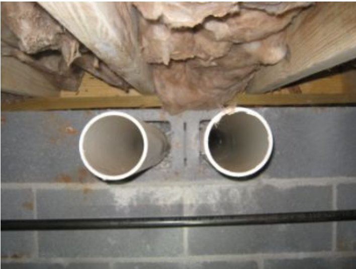
Rear crawl space vent at patio has been abandoned and suspect fungus was observed. Some crawl space vents are obstructed by concrete block and can not function. Properly correct crawl space ventilation as needed to protect structure.
