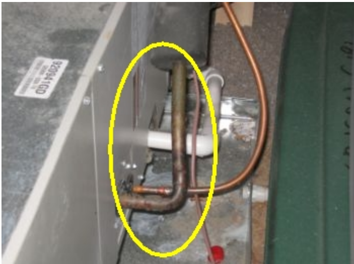
Cooling system refrigerant lines need insulation - Sections of the insulation on the compressor lines appear to be missing. These lines should be suitably insulated for the proper operation of the compressor.
