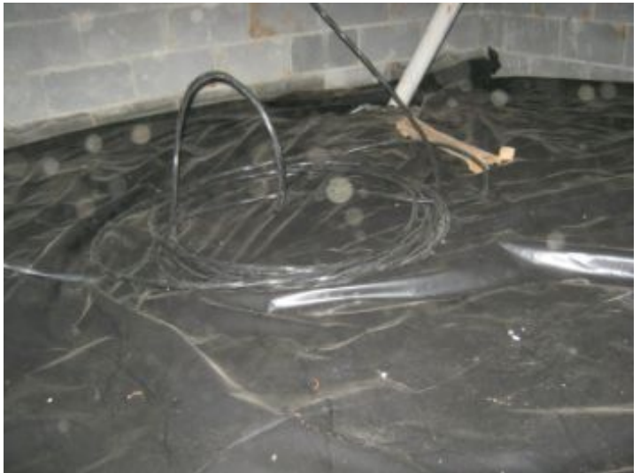
Unterminated wiring - Some wires viewed not terminated. Add wire nuts to all unterminated wiring in junction boxes/panel or otherwise properly terminate in junction box with cover as needed.
