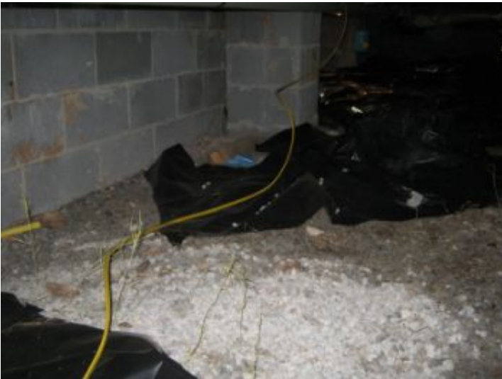
Wiring in crawl space is dangling and should be properly fastened in place to protect wiring from physical damage.
