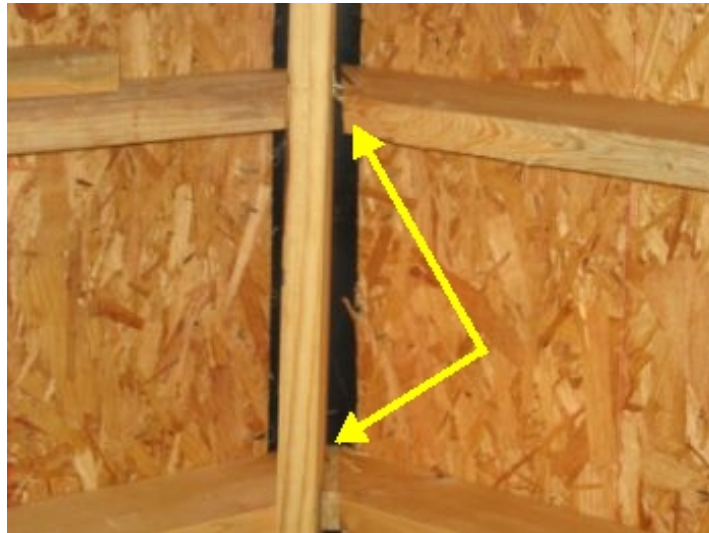
Top arrow shows large gap where rafter should meet ridge board, lower arrow shows shim where rafter should meet ridge board
