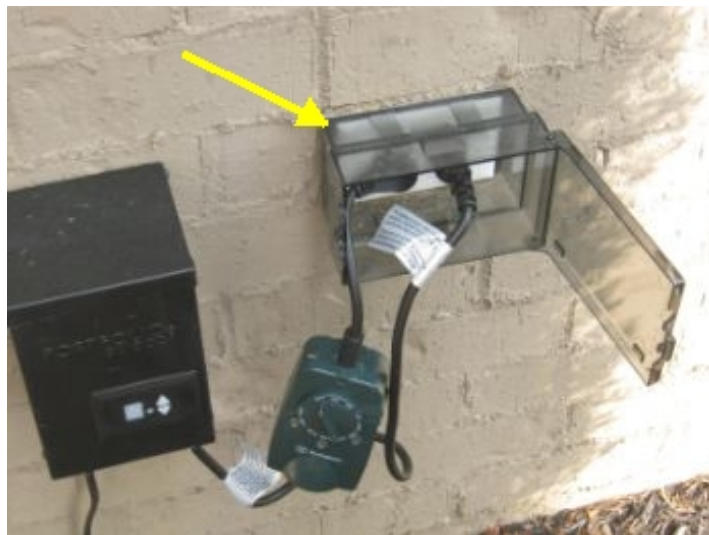
Periodic Maintenance Needed- Install proper continuous use cover at rear exterior receptacle
