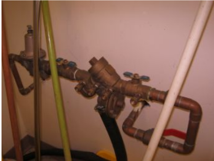
Back flow preventers require annual testing and reporting
