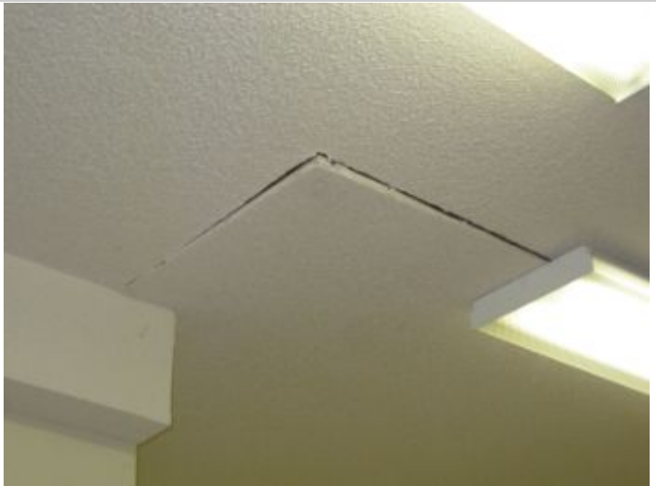
Damaged ceiling ready for correction at rear
