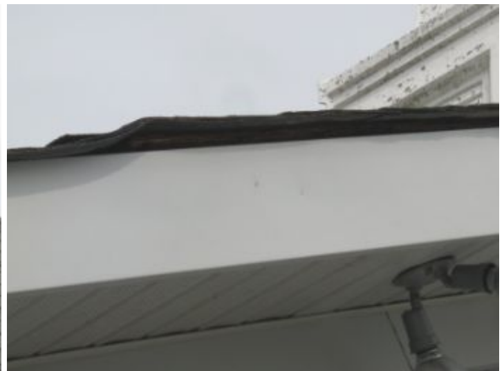
Some decking lifted
