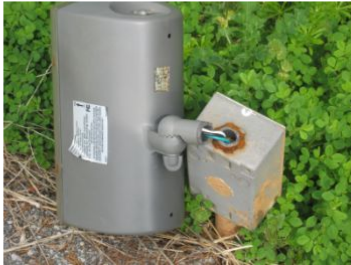
Damaged exterior lighting
