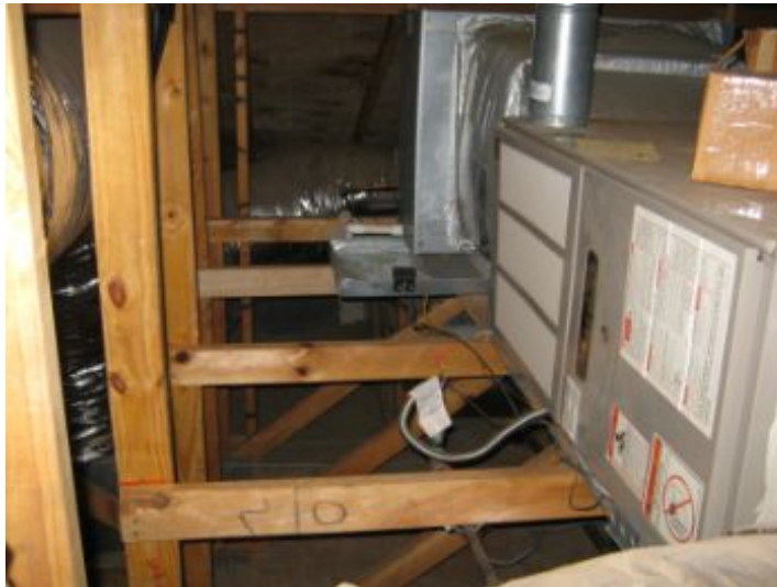
Trusses may not be designed for furnace platform attachment
