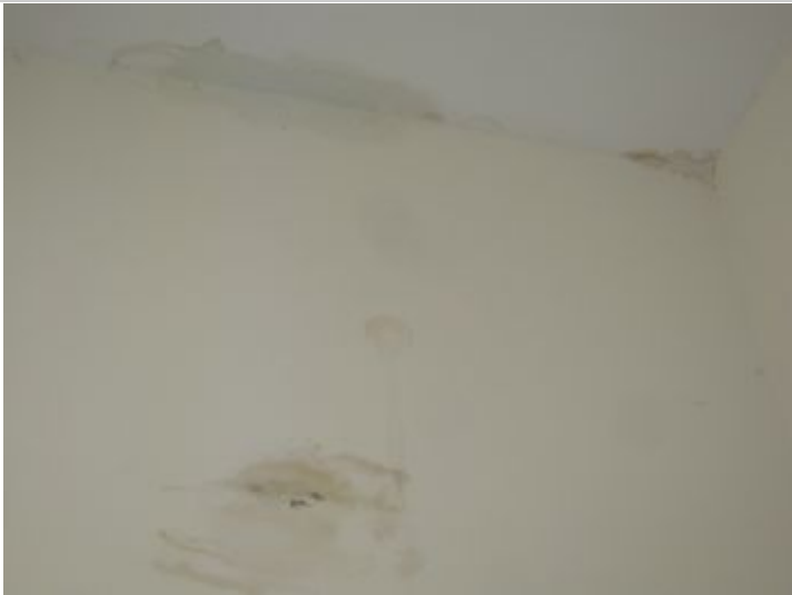
Ceiling and wall stains observed
