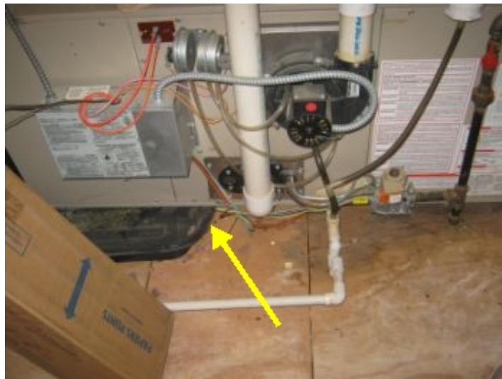
Upstairs office furnace overflow pan damaged and undersized
