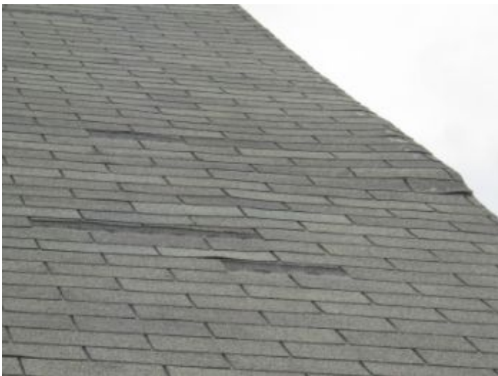
Representative roofing damage photo
