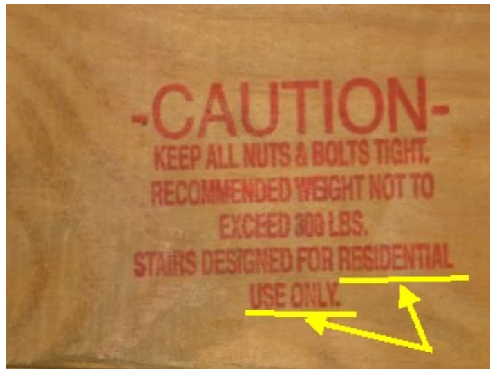
Attic steps not rated for commercial use
