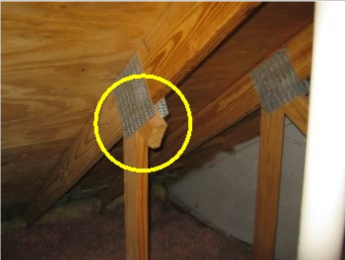
Unrepaired cut truss observed near upstairs furnace for office area
