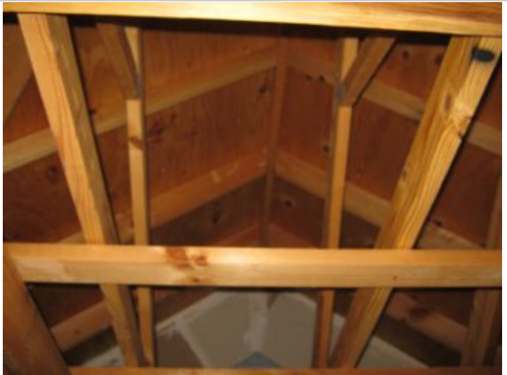
Some trusses appear to lack sheathing at rear attic area
