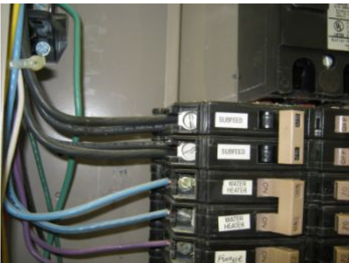
Double tap observed at front sub breaker panel
