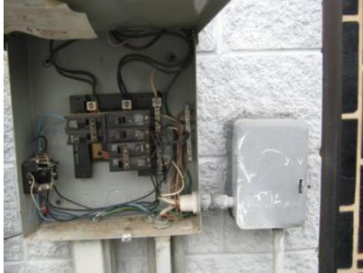
Improper wiring observed at left exterior AC disconnect panel
